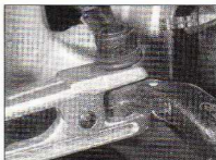
22.5 Release the track rod balljoint from the swivel hub using a universal balljoint separator
