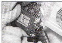
14.15e On models with electric windows, disconnect the wiring connector from the regulator as it is removed
