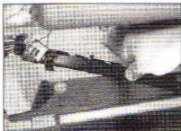
28.14a Release the retaining clips and ties, and free the wiring from the fascia metal frame . . .
