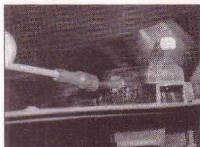
3.6 Disconnecting the intake air temperature control vacuum pipe from the air cleaner
