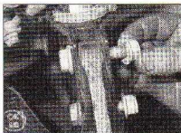
2.9 Unscrew the nuts and withdraw the bolts securing the suspension strut to the swivel hub
