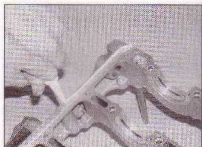
18.18 Apply a 2 mm diameter bead of silicone sealant to the outside of the groove (not in the groove itself), in the baseplate
