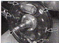
5.19 Apply a smear of anti-seize compound to the contact surfaces of the backplate (arrowed). Note the elastic band wrapped around the wheel cylinder
